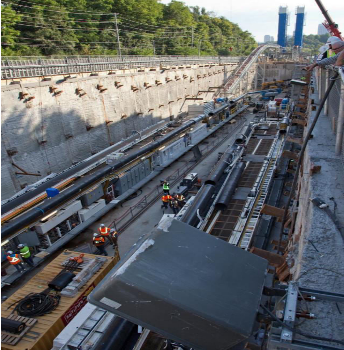
The launch shaft for the Crosstown LRT at Brentcliffe and Eglinton in 2015, image by Jack Landau
