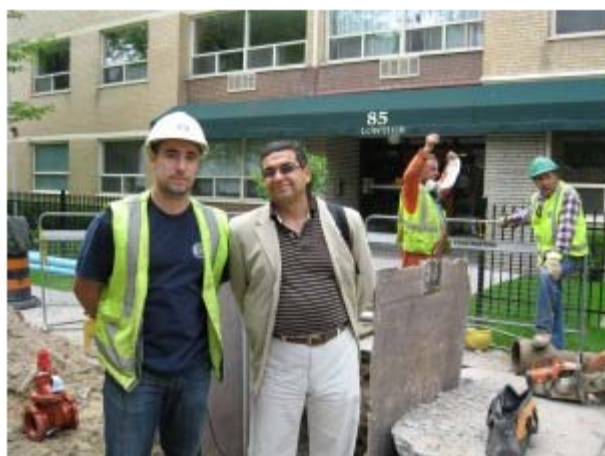
Frank Gazze (CG Construction Services) and Tamer El-Diraby (University of Toronto) stand near downtown Toronto watermain construction this morning.
